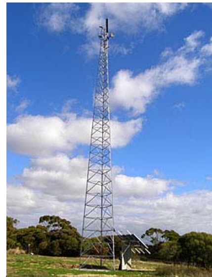
An Internode solar-powered WiMAX Base-Station site.
